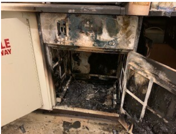
Pump cabinet at base of fume hood
